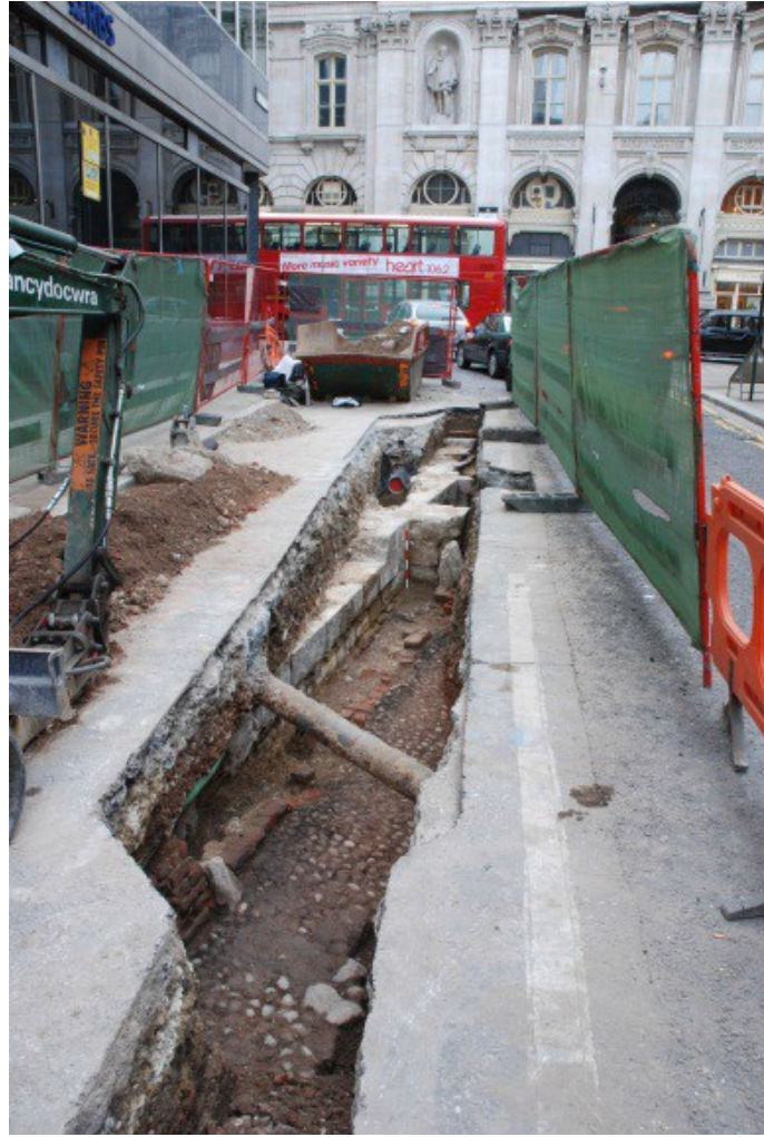
Figure 6: Buried structural remains of the Church of St Bartholomew the Exchange, Bartholomew Lane, City of London (Image: Compass Archaeology)
